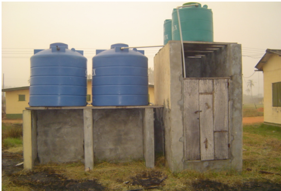
Plate 2: An Abandoned Borehole Fitted with Electrical Pump at Ebute-Lekki
