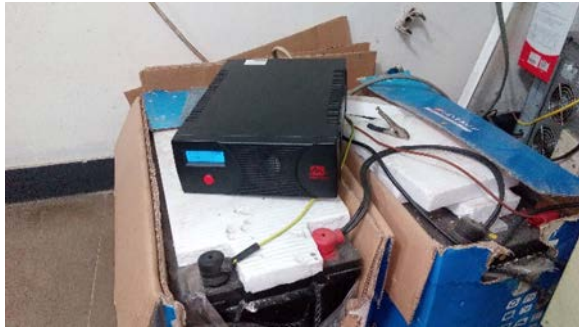
Figure 5: Batteries and inverter connected
